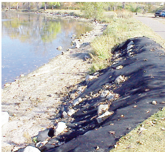
(ABOVE) In 2000, start of restoration along Lake Phalen in St. Paul. (RIGHT) View of the same site in 2002.
